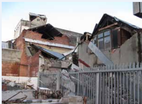
Figure 3.2: Failed gable end walls.
