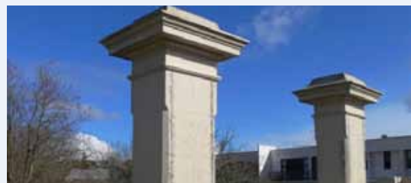
Figure 3.11: Vertical Near Surface Mounted (NSM) Fibre Reinforced Polymer (FRP) strip strengthening of chimneys.
