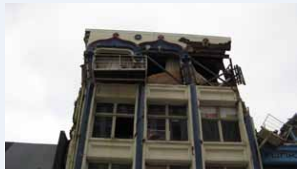
Figure 3.4: In-plane wall failure of piers on the top floor of a building.
