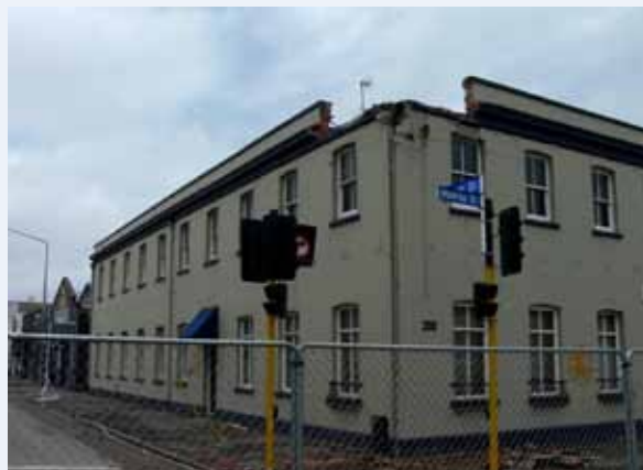
Figure 3.1: Failed parapet at the corner of a building.
