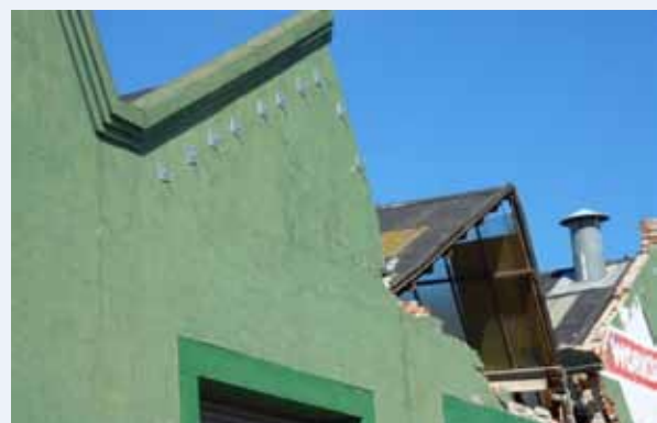
Figure 3.7: Example of a secured gable end that survived earthquake loading and a companion failed gable end that was not secured.
