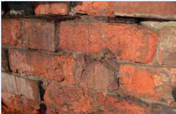
Figure 3.6: Severely degraded bricks and mortar due to the ingress of moisture into the wall.
