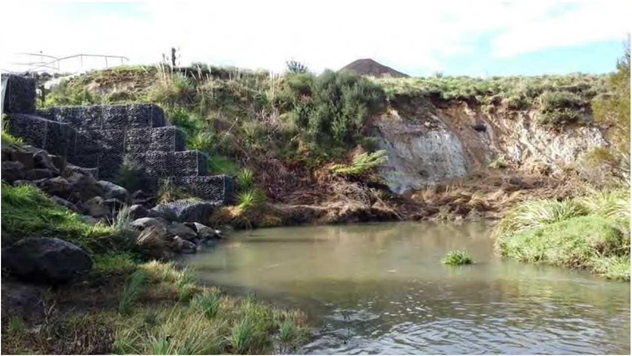
Figure 4: severe streambank slumping of the land parcel adjoining.
