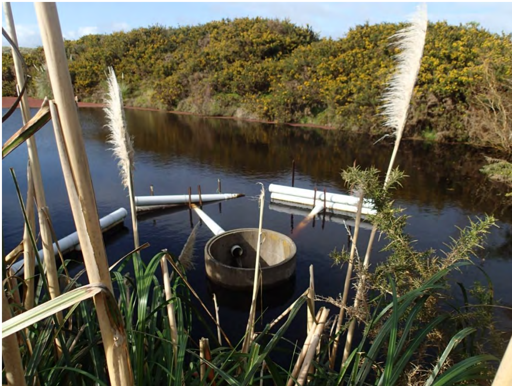
Photo 10. Decant structure from large on-line pond with vertical manhole and hanging pipes (providing a complete barrier to upstream fish passage).
