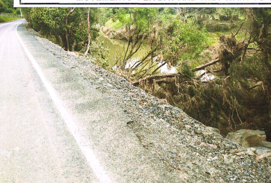
Gabian Baskets supporting Wall of Road
