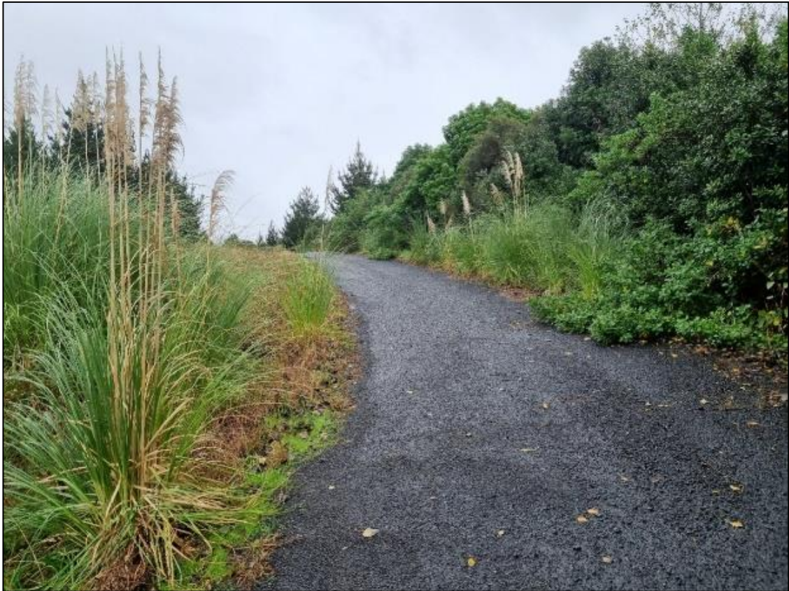
Figure 21. West facing view of overgrown vegetation and with sealed track extending through the central area
