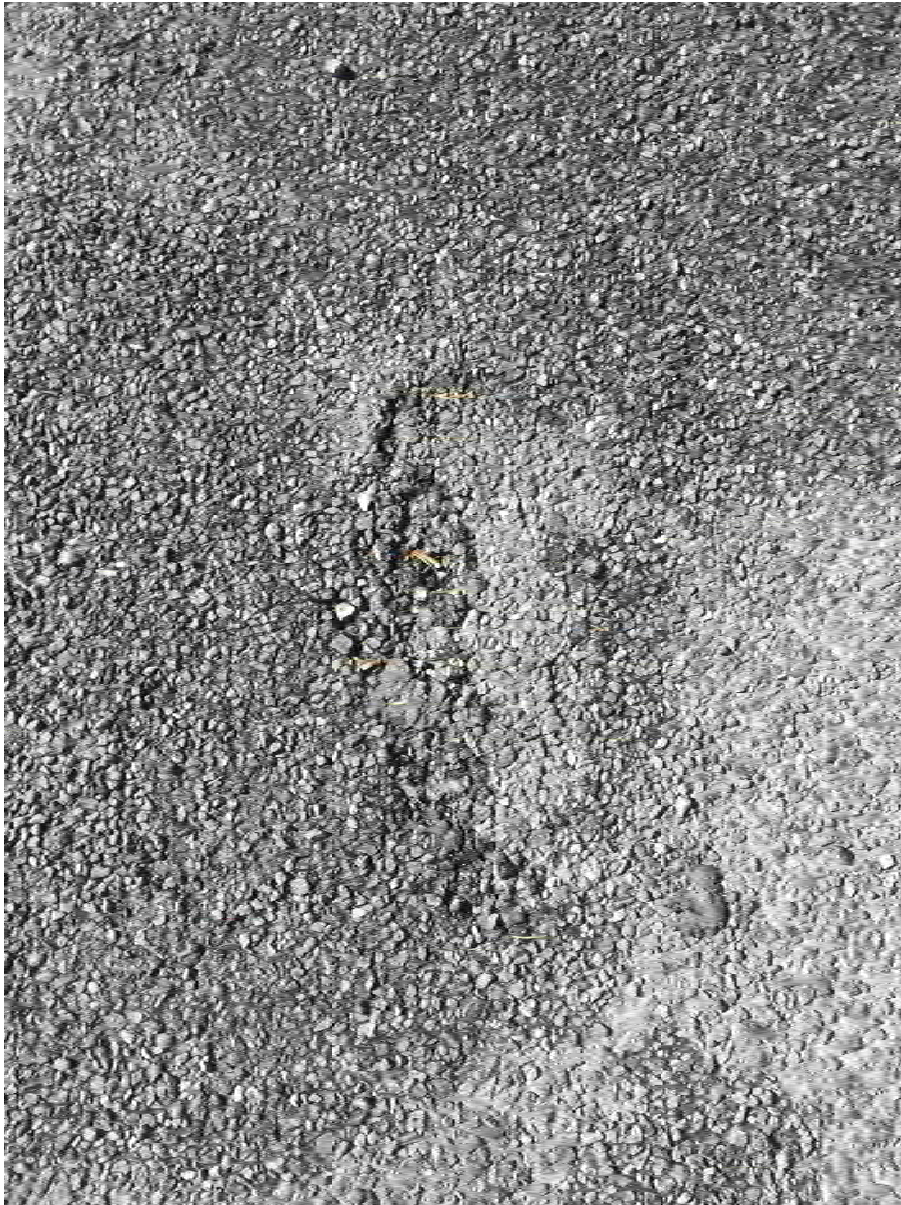
Damage to tar seal.
