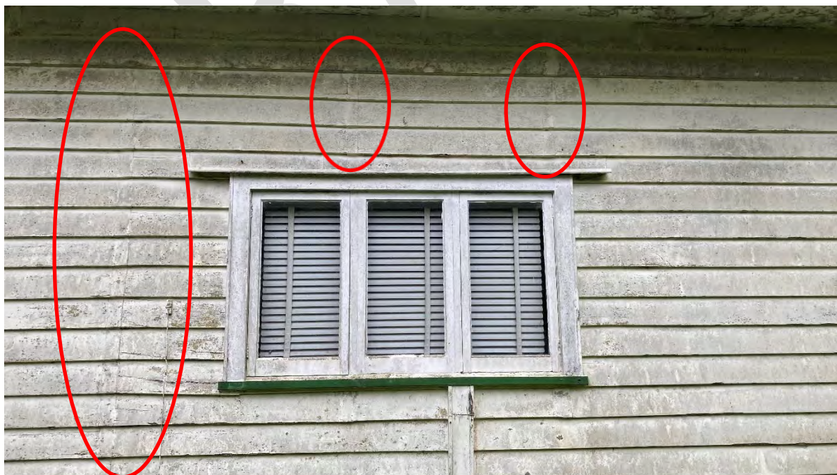
Figure 1. Left: Soakers covering transition between villa cladding and addition (later addition lies to left of image); Right: Double line of soakers covering joins in infilled sash window opening.
