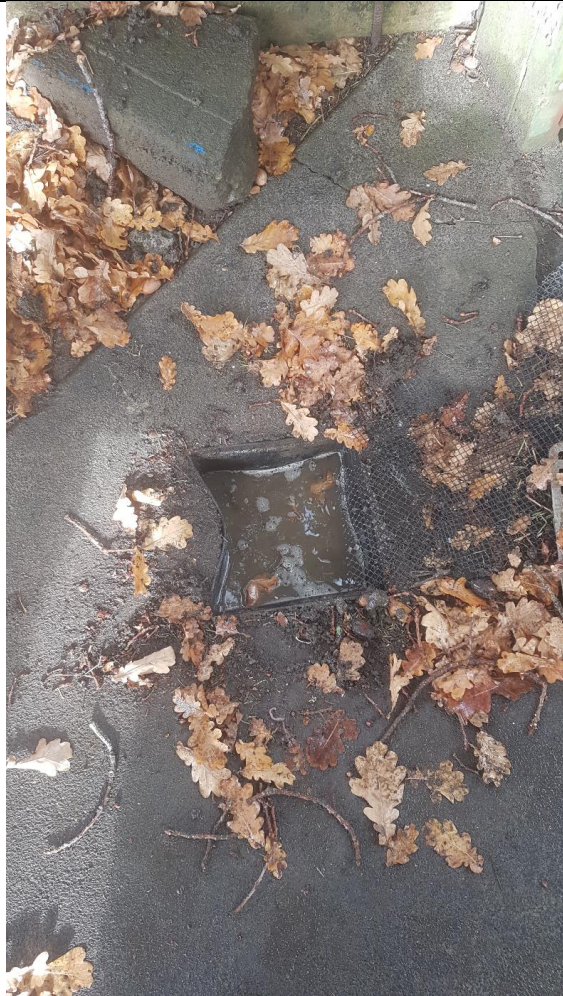
Drain system blockage from tree roots.
