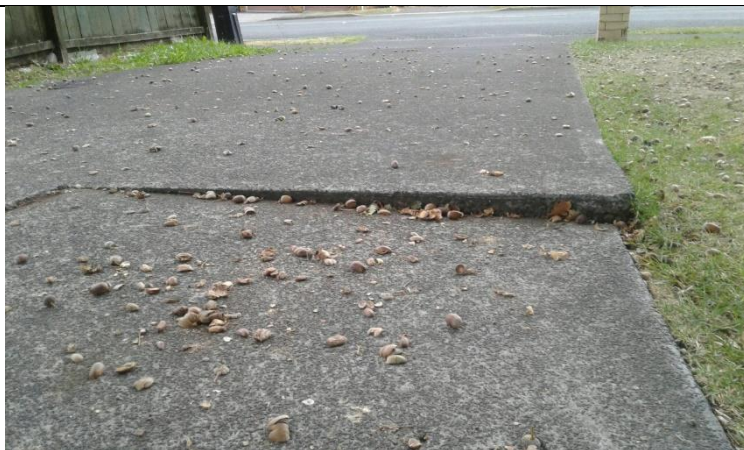
Driveway damage lifting and cracking.
