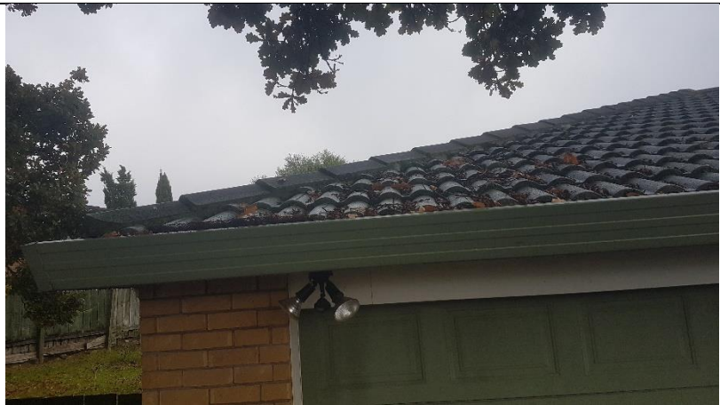
Leaves and debris on roof and gutter.
