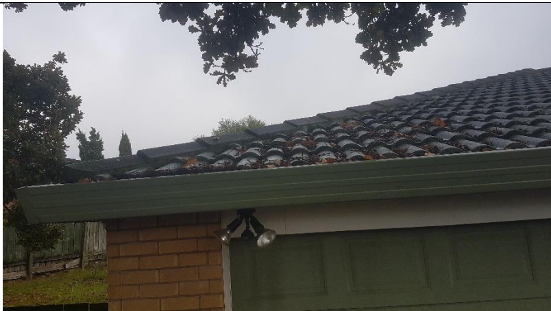
Leaves in roof and gutter from overhanging branches that are likely to cause blockage and damage.
