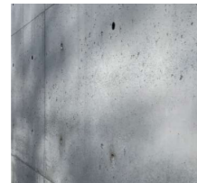
W.02 - Insitu Concrete Clear sealed insitu concrete lintels, sills and head beams.
