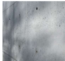
W.02 - Insitu Concrete Clear sealed insitu concrete lintels, sills and head beams.
