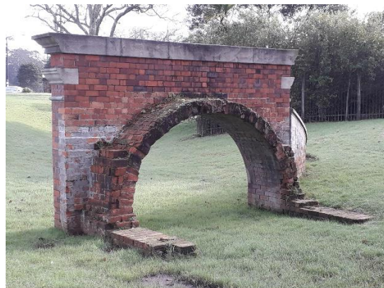
Figure 4: Rear view of Swan Arch showing the truncated vault structure with lower walls still present. In the background is the fenced-off vault.
