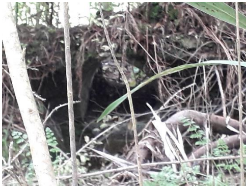
Figure 5: Part of the remaining vault structure with what appears to be a window to the west wall.
