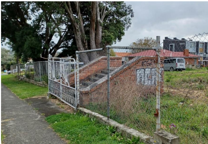
Figure 7 and Figure 8: Steps to the former Sunday school hall (Auckland Council, May 2022).
