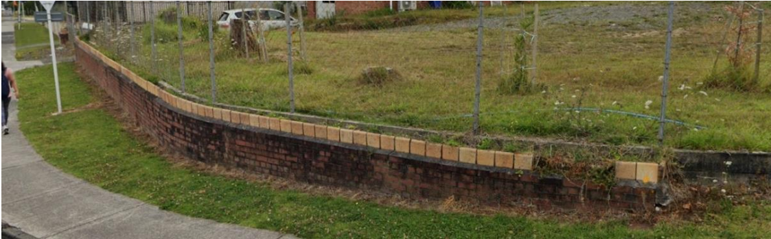
Figure 5: The remains of the boundary retaining wall (Google Street View, 2021).
