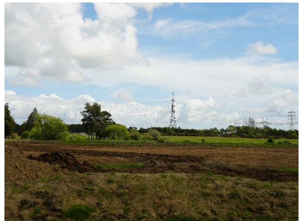
Figure 4-4: Earthworks in greenfield development – Drury South Crossing, Quarry Road (image: Aurecon, Oct. 2023)
