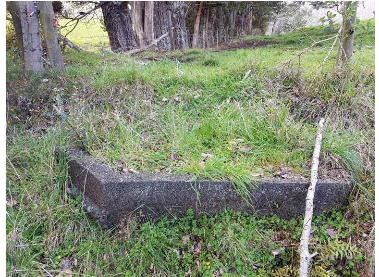
Concrete Stream Stopbank
