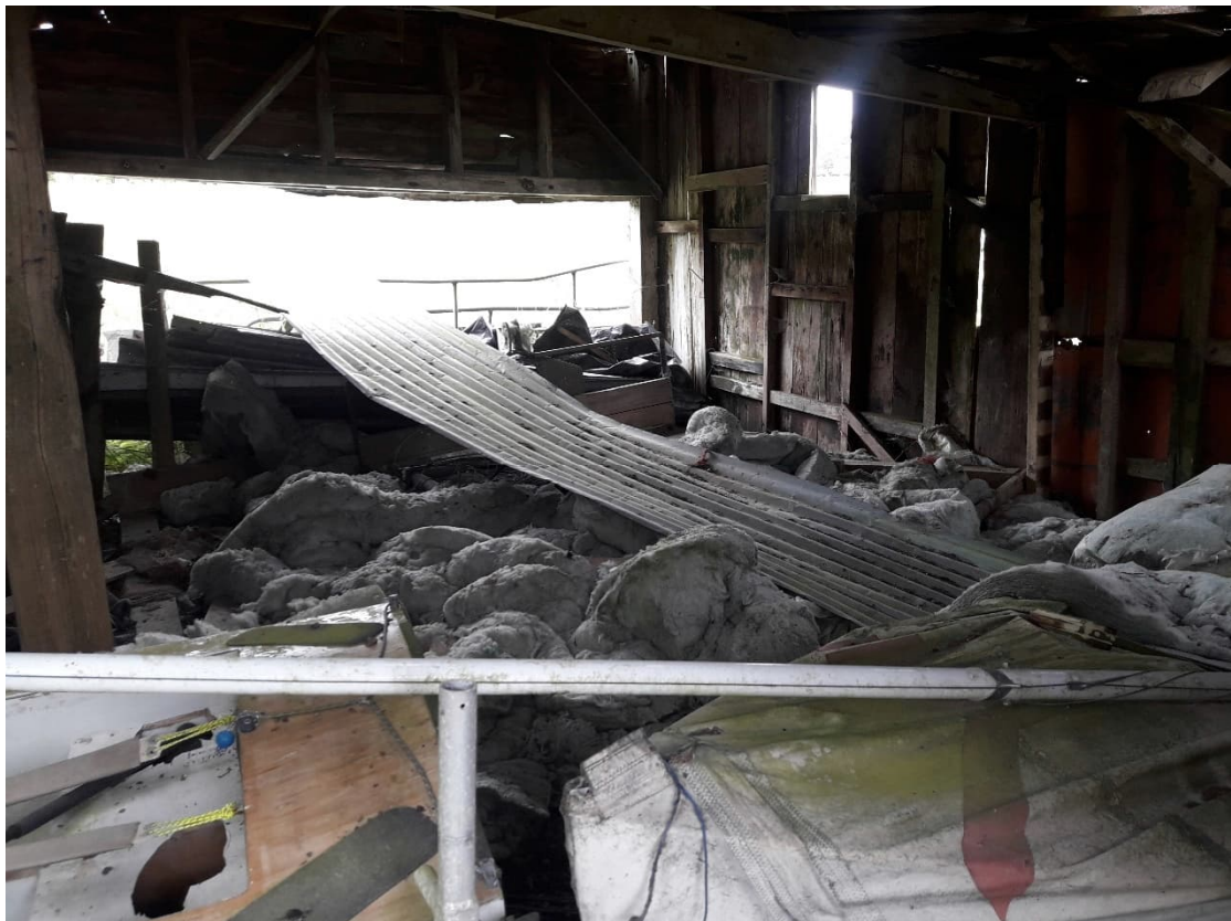
Figure 33: Dilapidated storage shed, timber storage and other unknown items.
