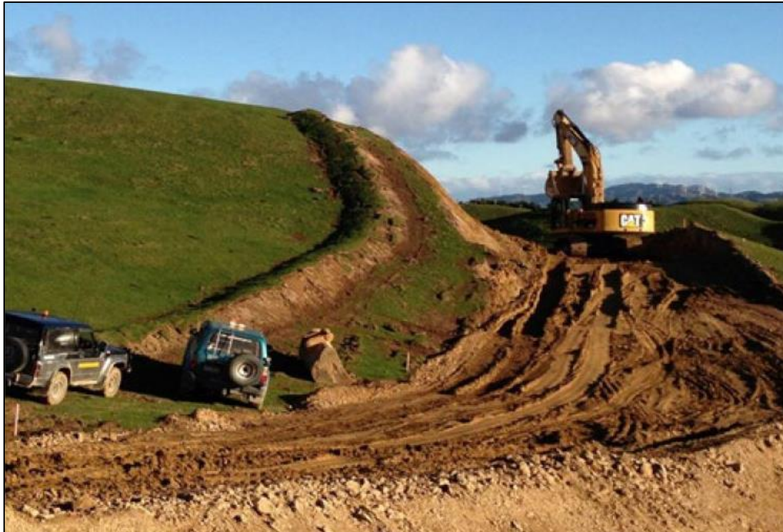
Figure 8: Photograph of Clean Water Diversion Bund
