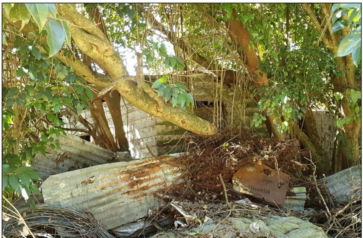
Figure 37. Substantial sized tree growing out of a window of the structure with building and other waste seen piled up around it
