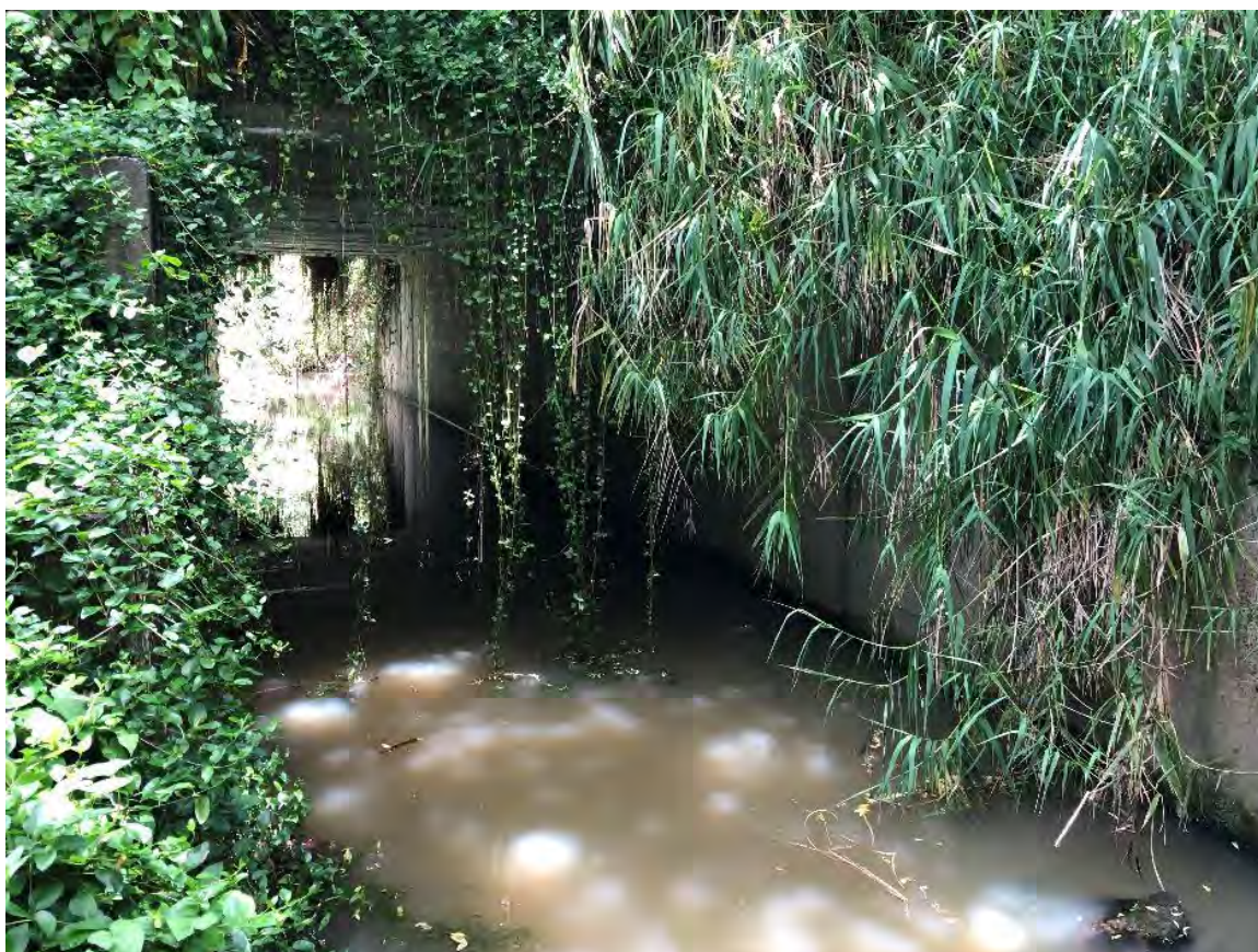
Figure 10-2 Under sized Waiarohia culvert
