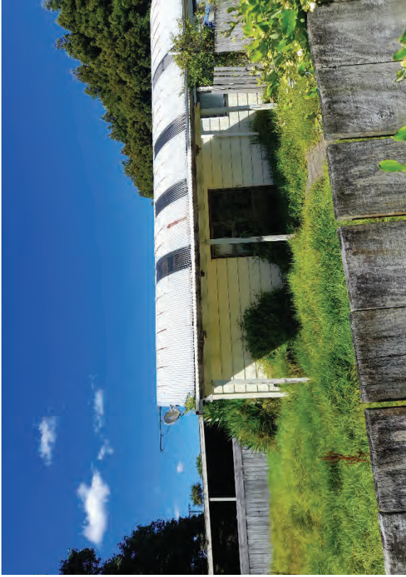
Photo 5: View from the associated structure in the south-west corner of 51 Lathrope Road, the structure contains what appears to have been a site office / admin facility and implement sheds for equipment and other sheds for use unknown.
