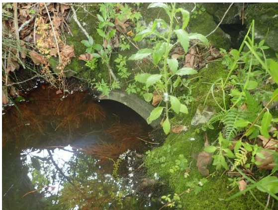
Photo 3. 2 – water entered via a culvert under SH1.
