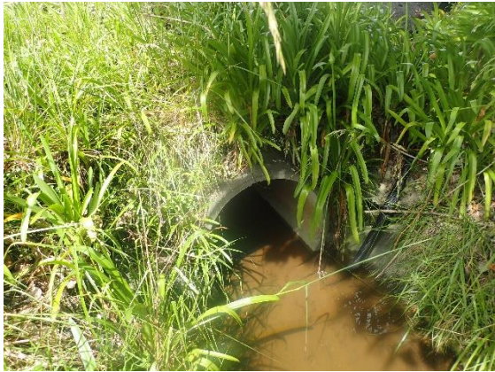
Photo 1. 1 – water entered via a culvert under Valerie Close.
