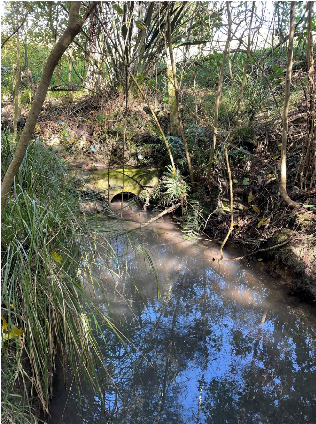
Figure 1 Undocumented Outlet to Stream
