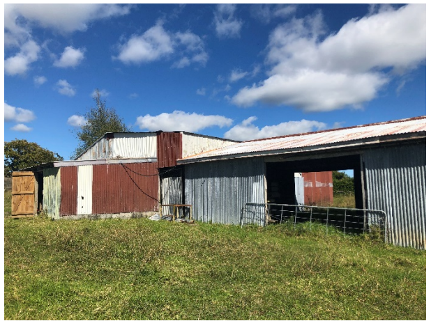
Photo 28: Closer view of building associated with stock yards in south-eastern portion of the site.
