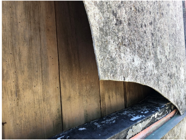
Photo 19: Close up of exterior of building in south-western portion of the site, showing potential ACM.
