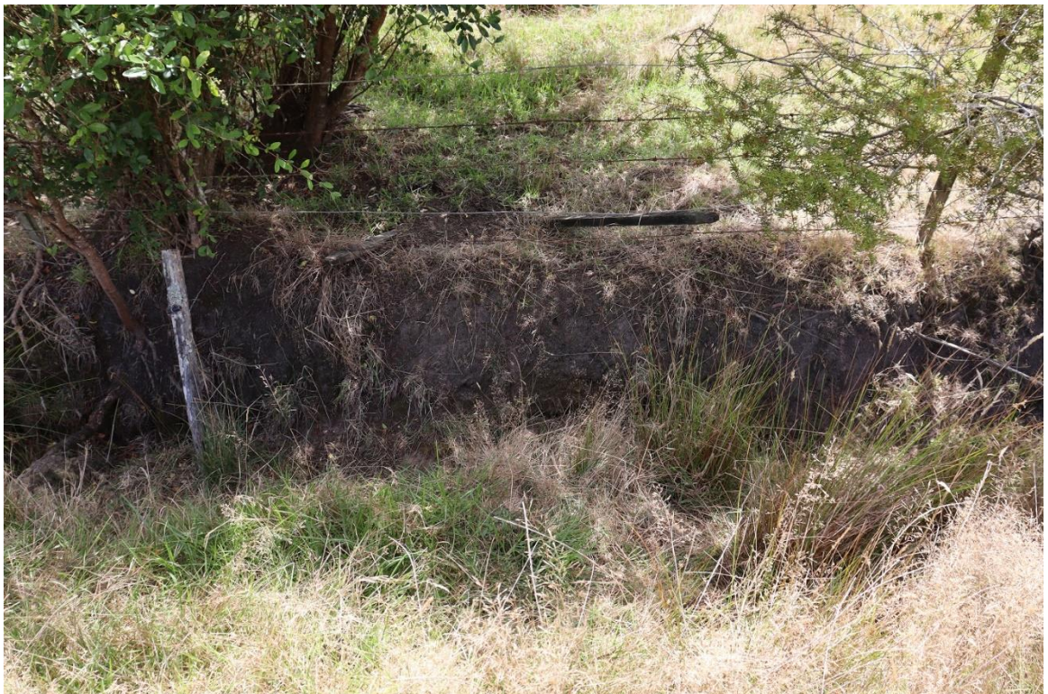
Figure 18. Stream running through Lot 2 DP 481942 showing erosion. Facing northeast
