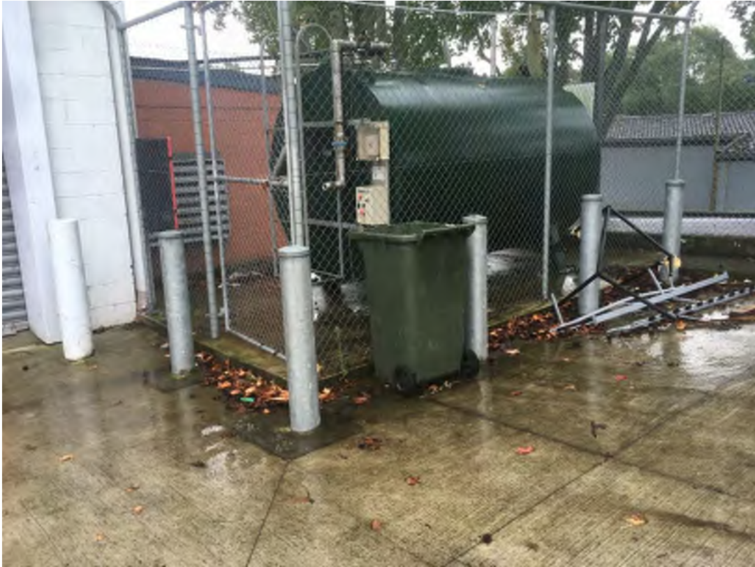
Photo 2: The un-bunded above ground storage tank.
