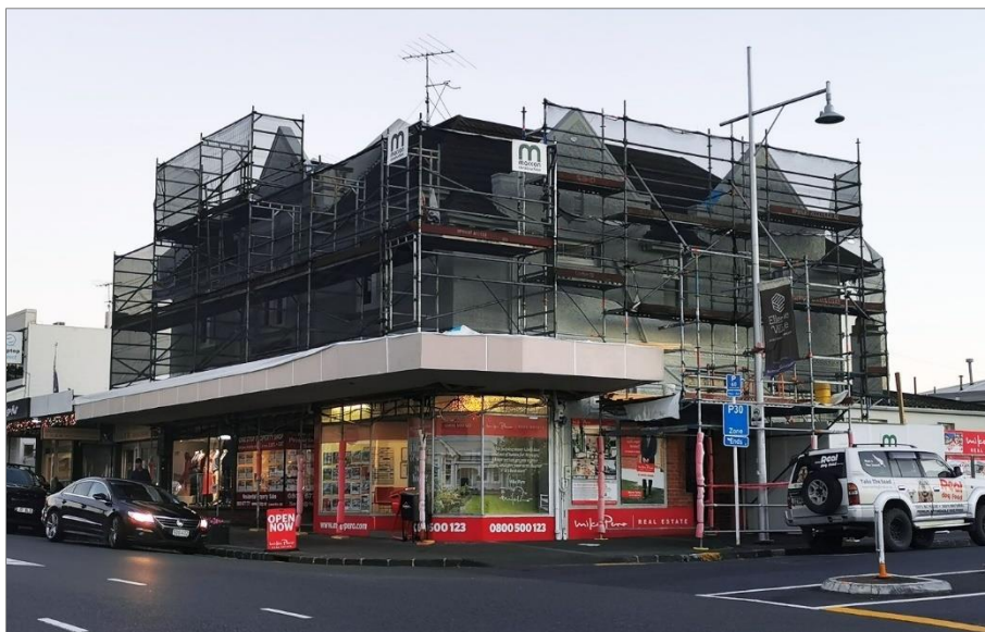
Figure 27 (top): The shopfronts on the corner of Main Highway and Ladies Mile. Figure 28 (middle): The corner shopfront and the entrance door to the three-bedroom flat on Ladies Mile. Figure 29 (bottom): The corner elevation of the building taken in May 2022, showing the nearly finished new/replacement verandah.
