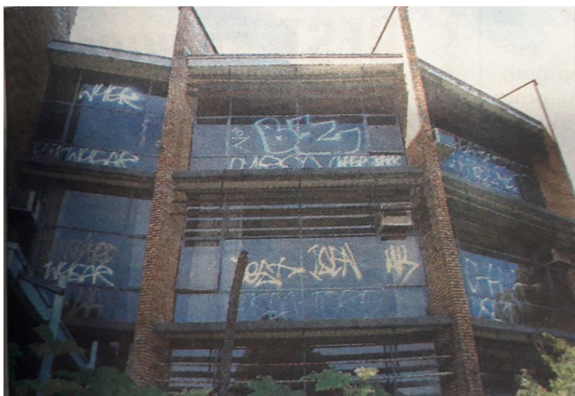
Figure 7. The building in January 2003 showing its derelict state. 44
