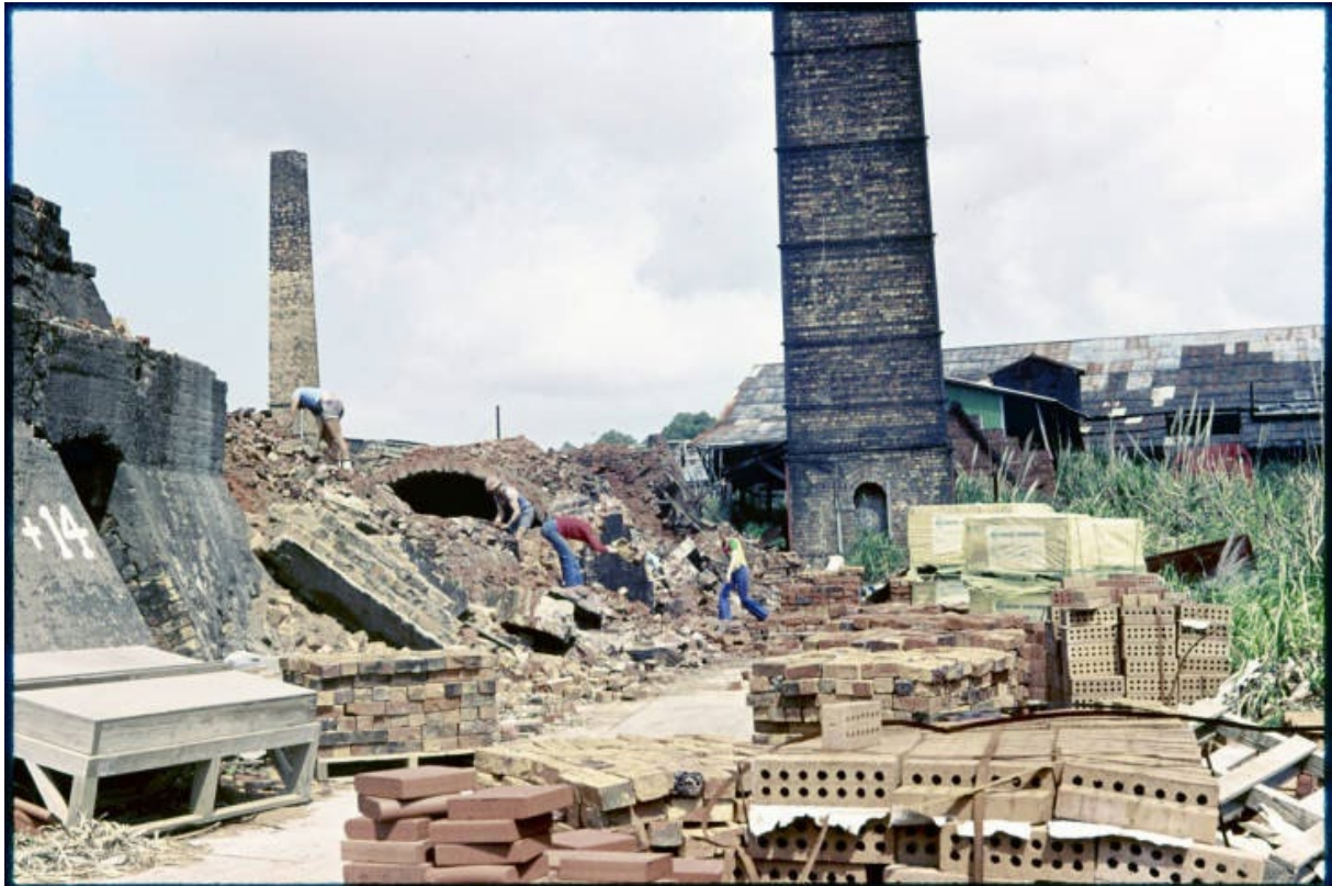
Figure 27. View of scene soon after the start of the demolition period at the former Gardner works, part of the Amalgamated Brick and Pipe Company's works, north side, showing the smoke stacks for the engine shed and for the kiln. Taken in December 1978 by J. Diamond. 115
