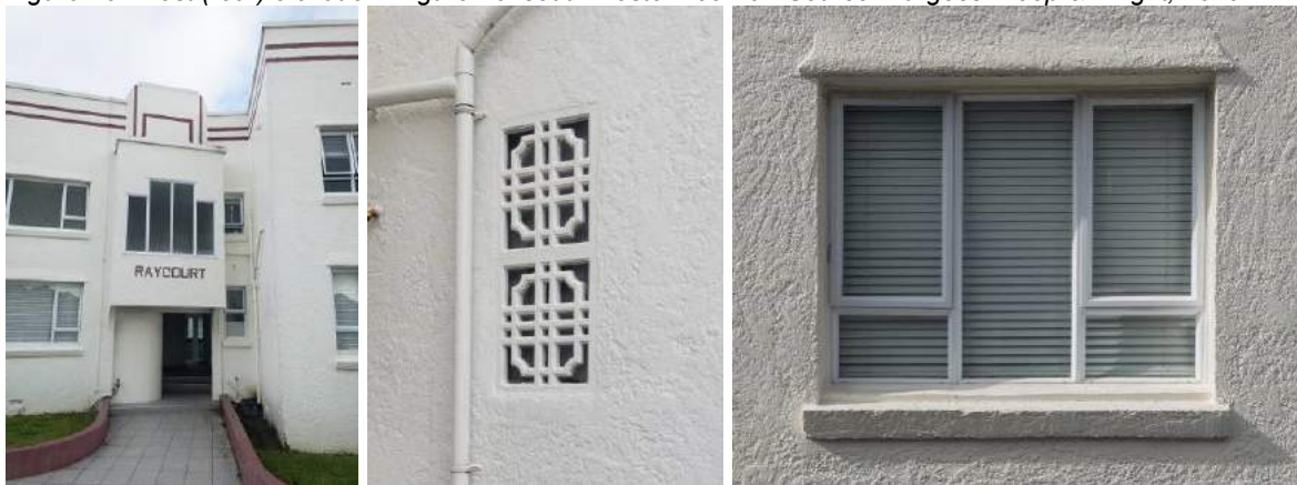
Figure 17: Main entrance. Figure 18: Decorative brick vents. Figure 19: aluminium joinery (replacement) and rendered masonry in skip trowel texture. Source: Burgess Treep & Knight, 2019.
