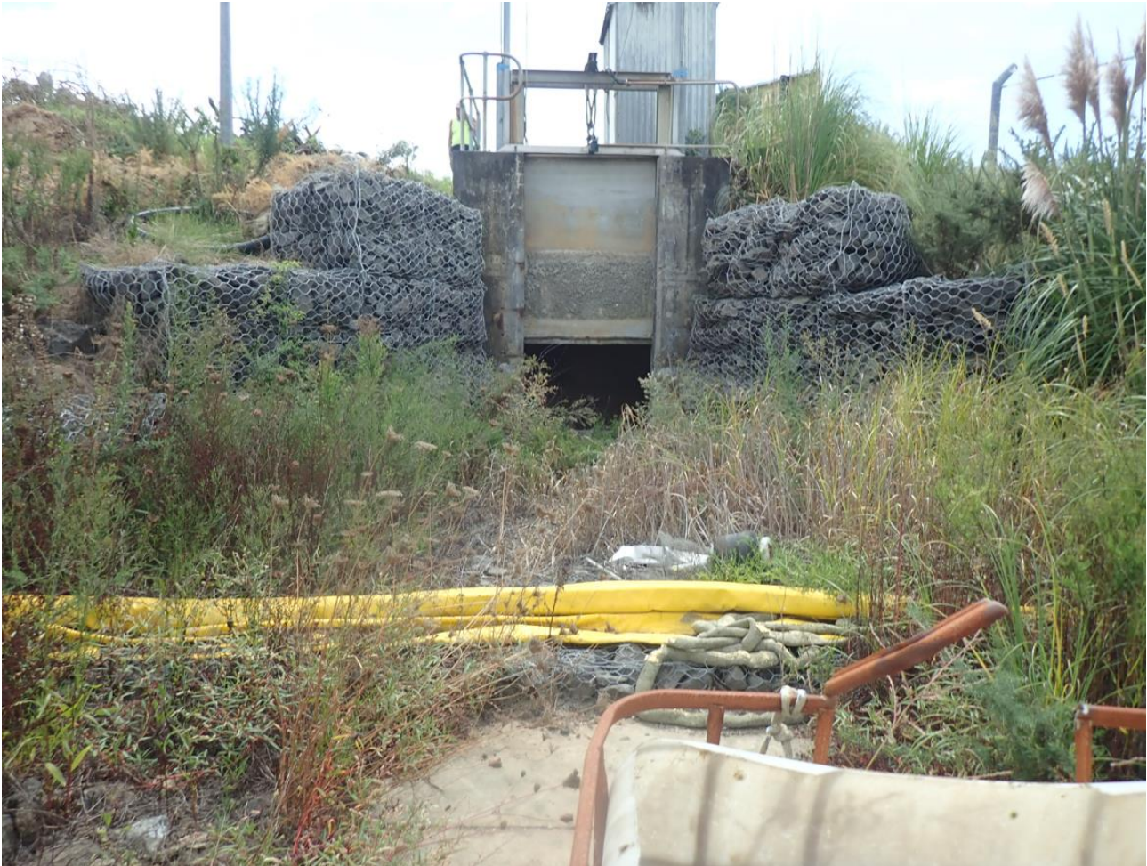
Figure 11: Floodgate at the water-cooling pond outlet
