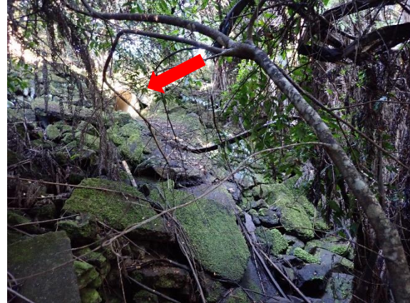
Photograph 3.2: Perched culvert (indicated by the red arrow) is located at the downstream end of the catchment (refer Site N1 on Figure 2) and would limit fish movement into the Northern Stream system.
