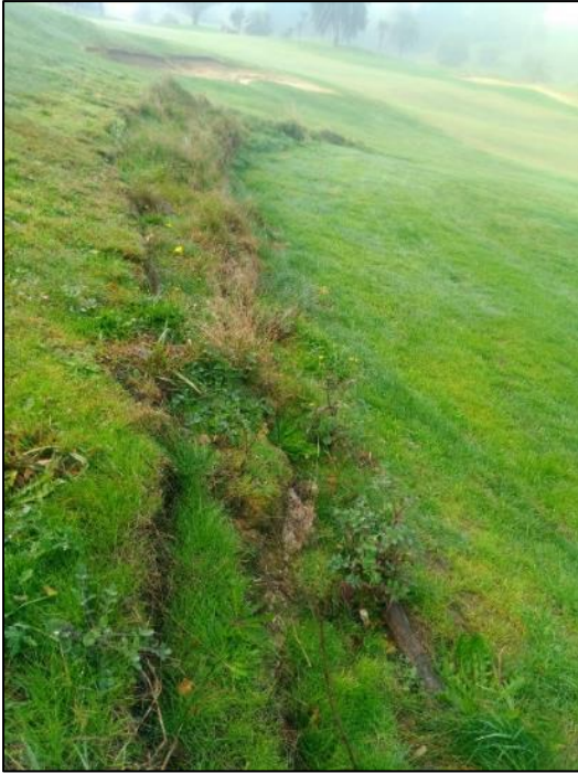
Figure 7: Toe of instability near Jack Lachlan Drive
