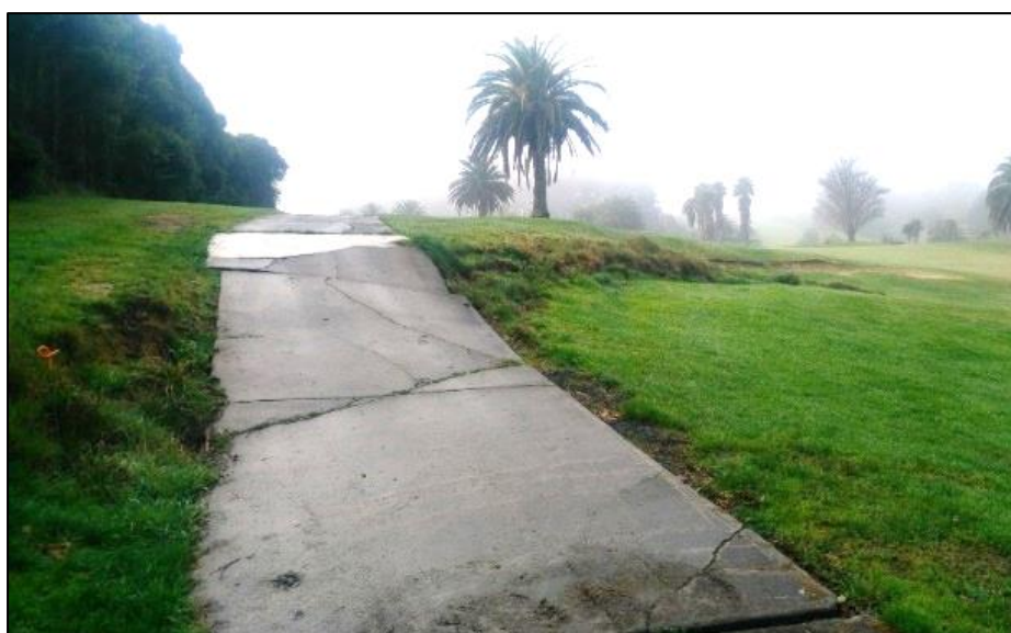
Figure 6: Headscarp of instability adjacent to Jack Lachlan Drive
