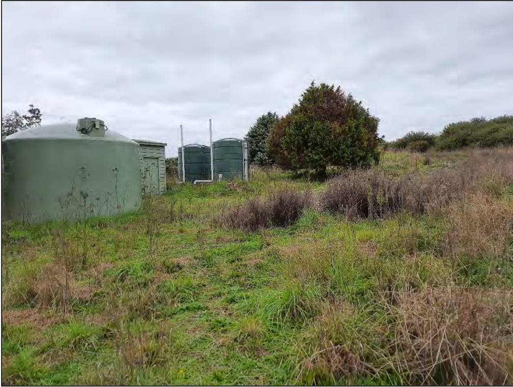
Photograph Appendix B.5: Looking north/north-west, the Formosa wastewater treatment system which comprises of a series of concrete settling tanks was observed towards the centre of the golf course. Control room and above ground tanks observed in the photo.
