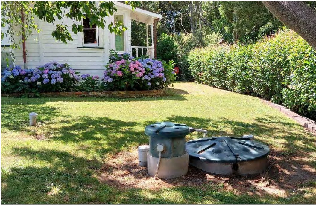
Photograph Appendix B.21: View east of inground septic tank system.
