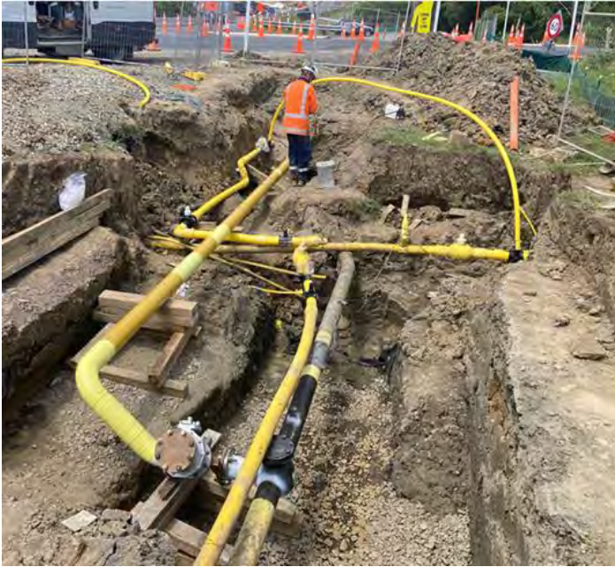
Gas diversion at Berrys Bridge
