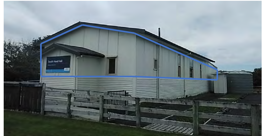
Above: cladding containing asbestos
