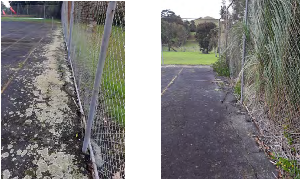
Below: Previous failing hardcourt and fencing
