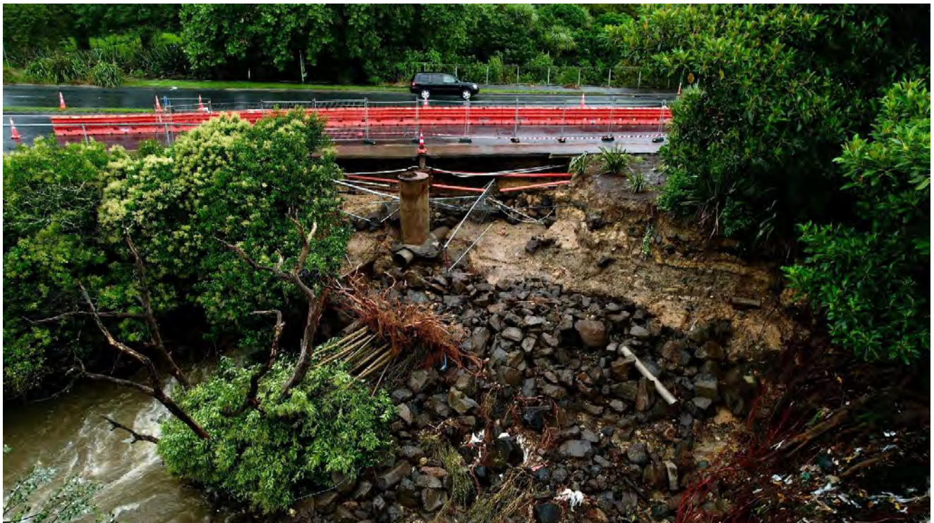
Damage to culvert on Great North Road
