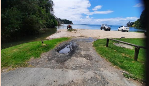
Sandys Parade – water pipe leak
