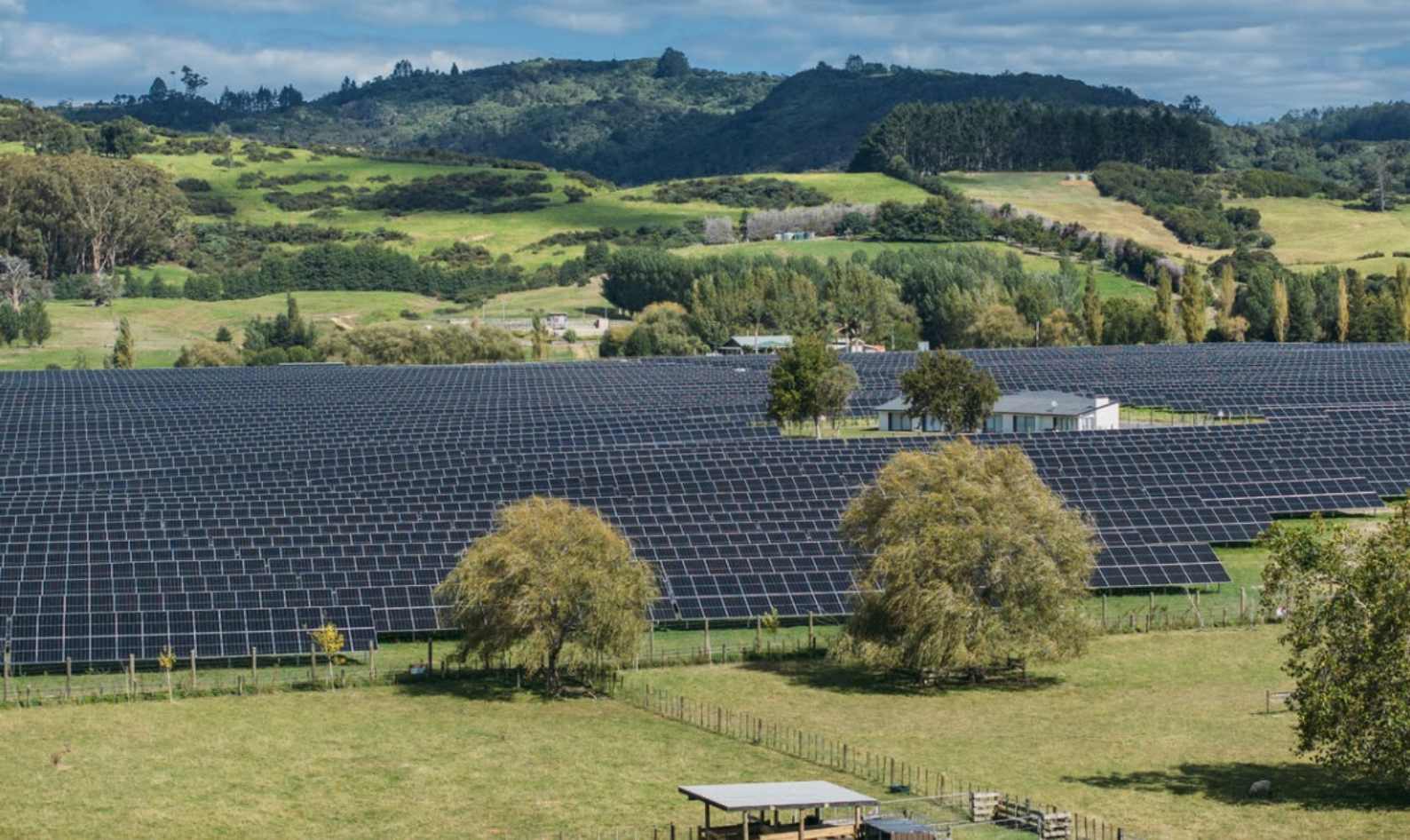
Solar farm at Ardmore.
