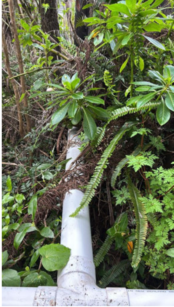
Picture 22: 4 Subsoil exit into dense bush (2)
