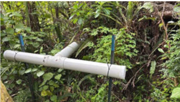
Picture 23: 4 Subsoil exit into dense bush
