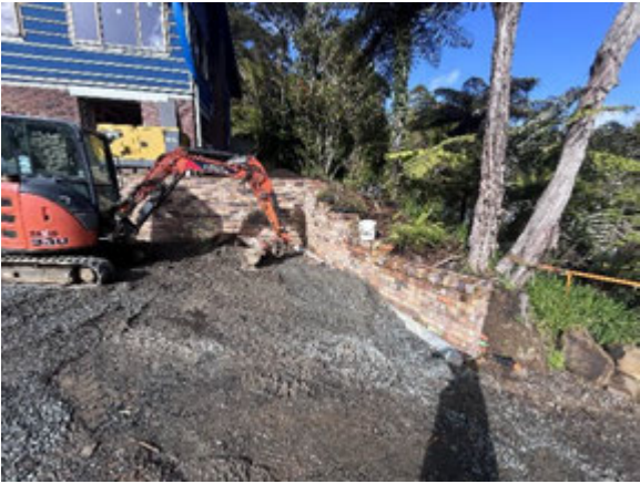
Picture 1: Current driveway gravel area (2)
