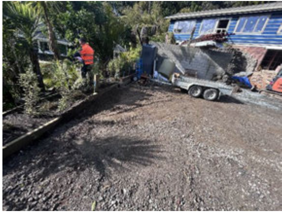
Picture 2: Current driveway gravel area
