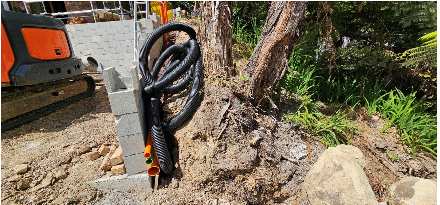
Figure 3: Mature kanuka with extensive root severance present.
