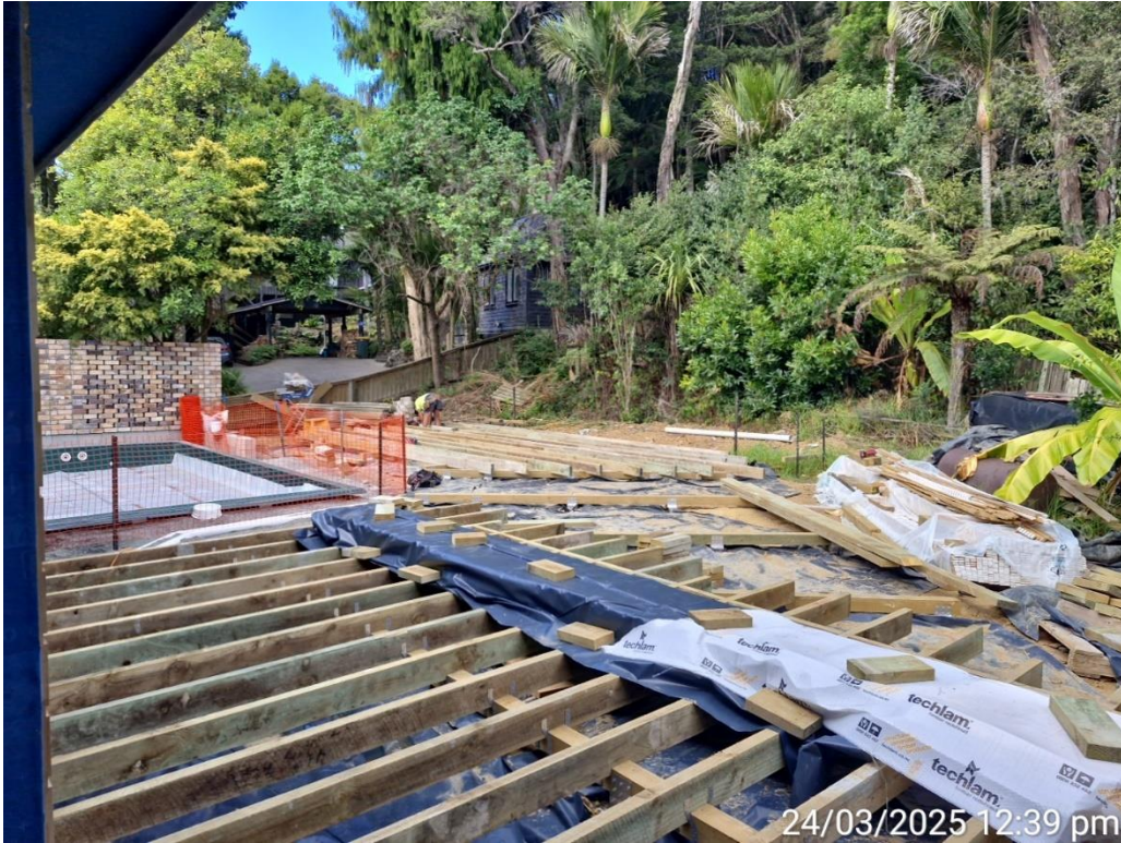
Figure 3: looking at rear at house where pool, minor dwelling and rear deck is under construction.
