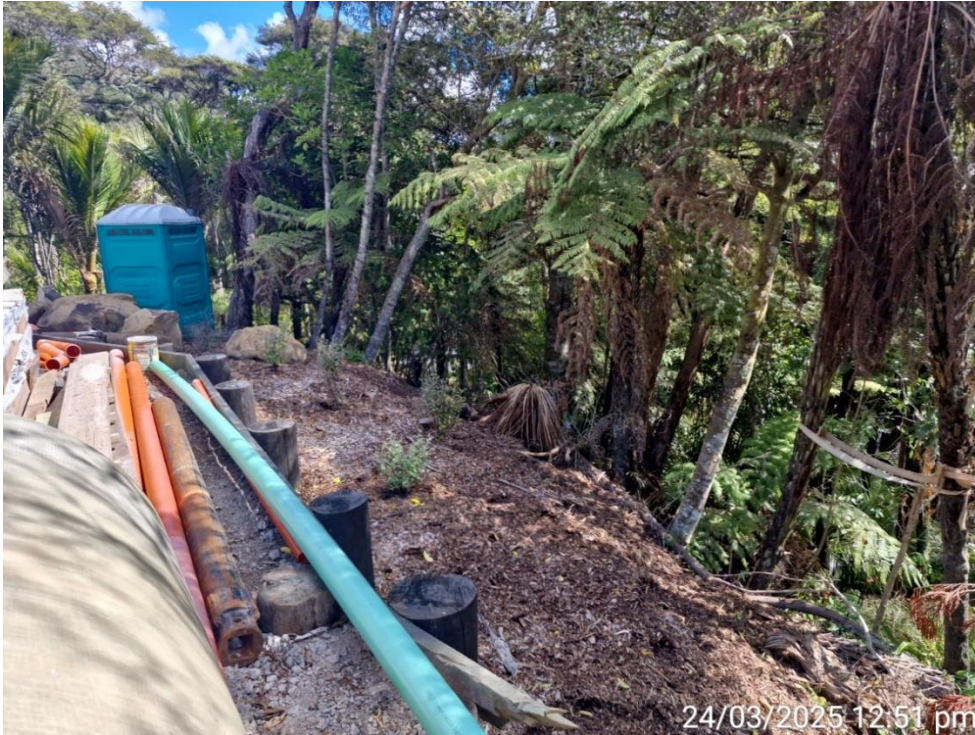
Figure 7: looking north-eastern side of property and SEA, new retaining wall and area where T-Bar and riprap will disperse stormwater. Native forest seen on slope will be covenanted.
