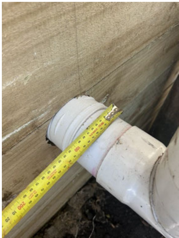
Picture 8: Higher tank orifice size which is to be verified by contractor to ensure 20mm diameter orifice.
