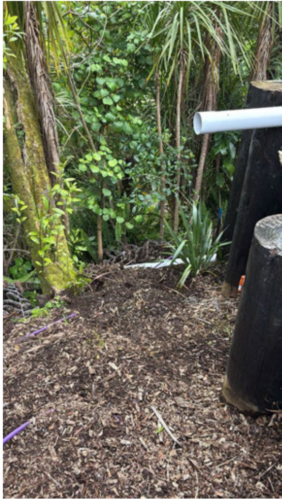
Picture 20: 3 Subsoil pipe extensions into dense vegetation (3)
