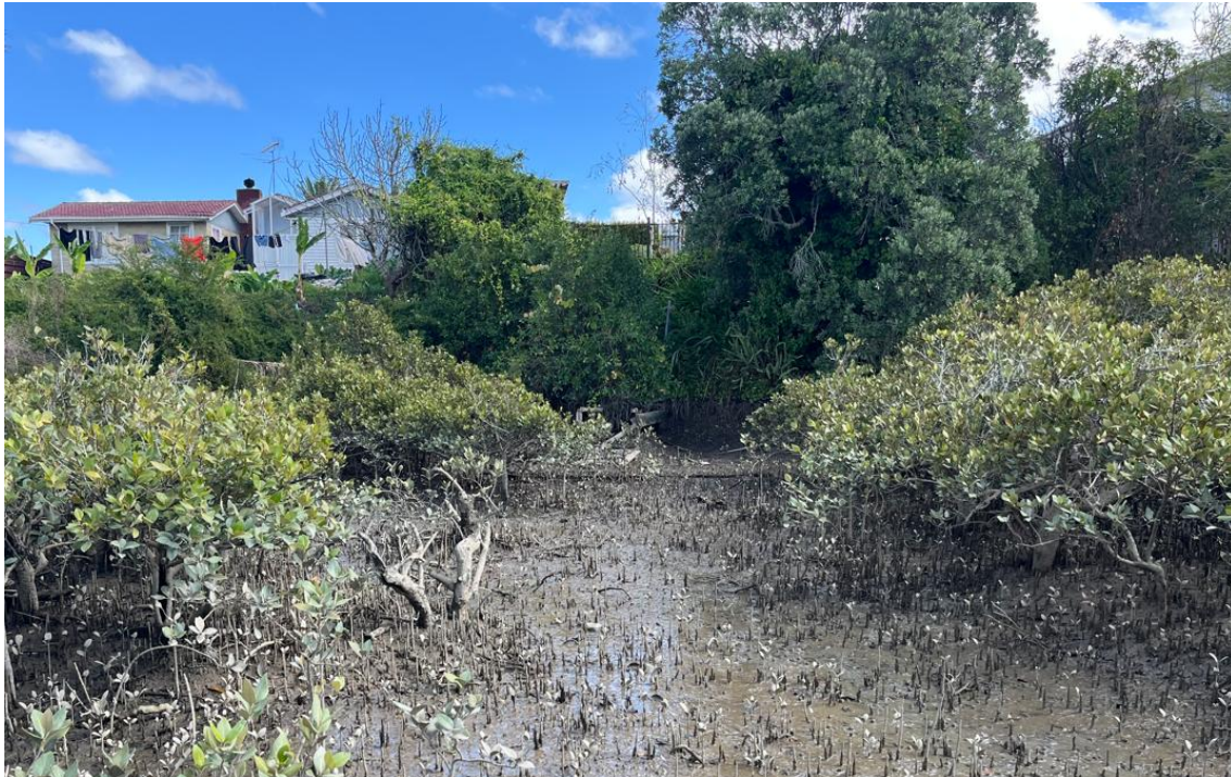
Figure 7: Vegetated bank and exposed substrate at the toe of the slope (153 Edgewater Drive).
