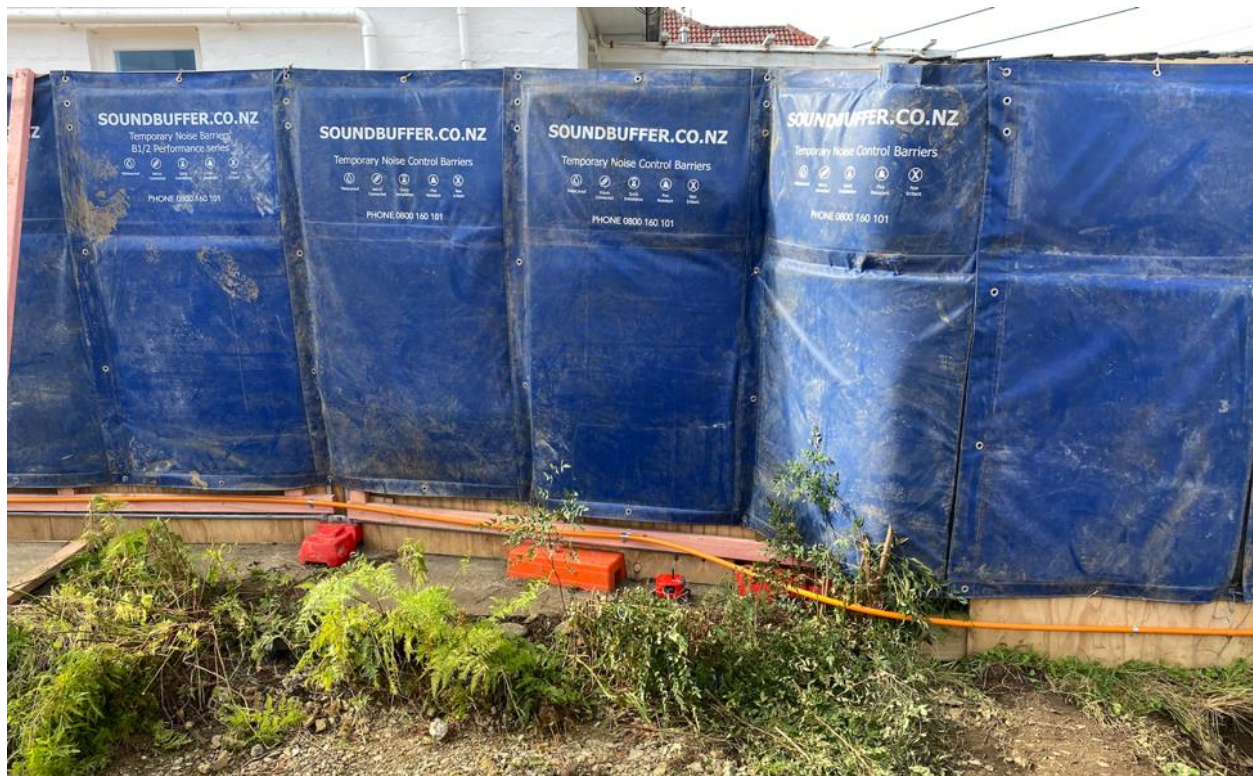
Figure 10 - Example of Acoustic blankets affixed to existing landscape fences
