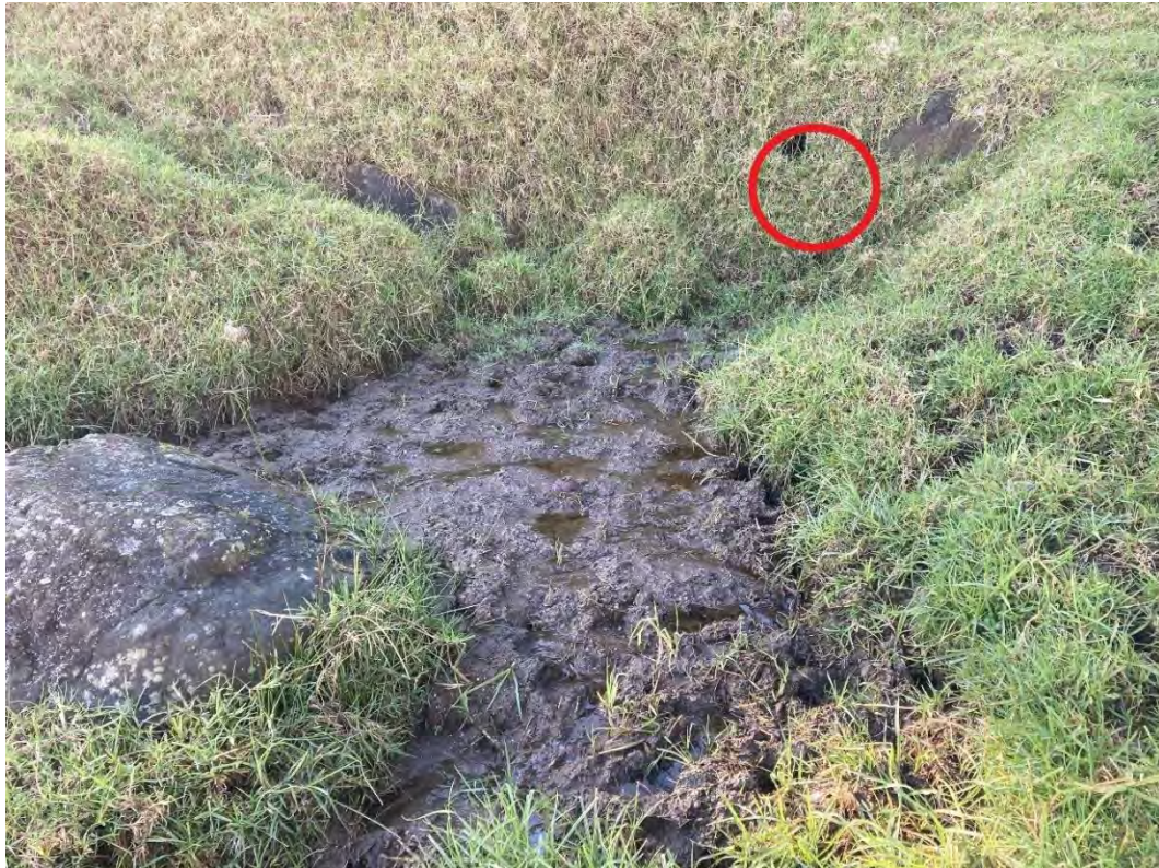
Plate 39: Heavy pugging in intermittent stream proposed to be enclosed within a culvert below the old quarry. Pugging has created a thick layer of very wet mud with no habitat value for indigenous fish. Red circle indicates approximate location of existing culvert discharge point. 12 August 2021.
