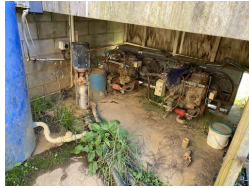
Milking shed pumps – location 11
