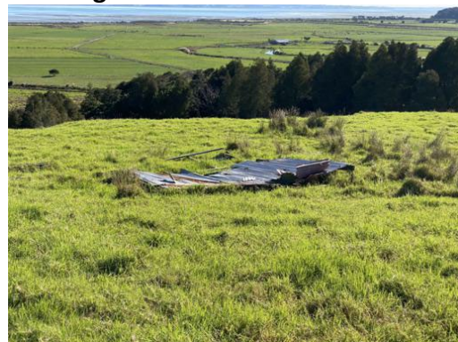
Collapsed shed – location 27
