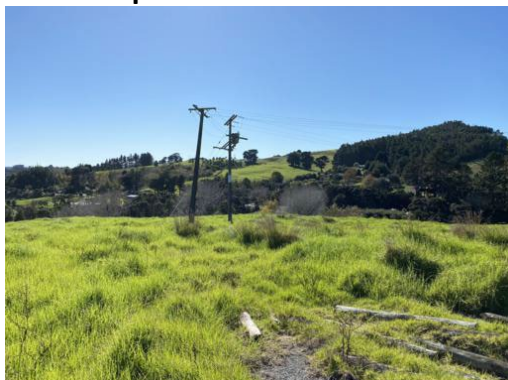
Pad & transformer – location 8
