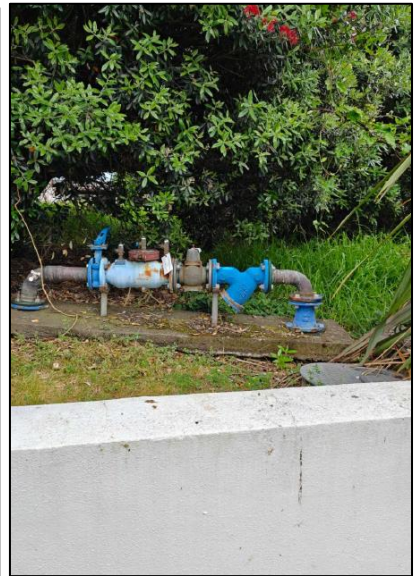
Watermeter M01A096864 for fire sprinkler
