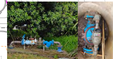
EXISTING WATER METER AND BACKFLOW PREVENTER FOR FIRE SPRINKLER TO BE RETAINED AND RELOCATED FOR PROPOSED DEVELOPMENT
