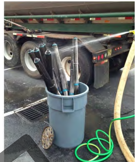
Rinsing of dirty filter cartridge tentacles with a low-pressure garden hose sprayer and using a plastic garbage container to capture rinse water.
