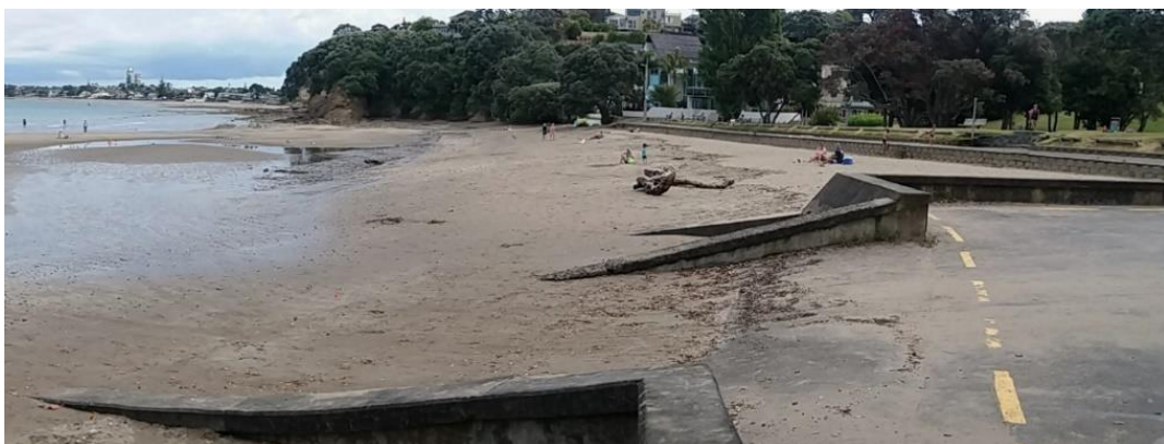
Figure 16: Castor Bay Beach and boat ramp
