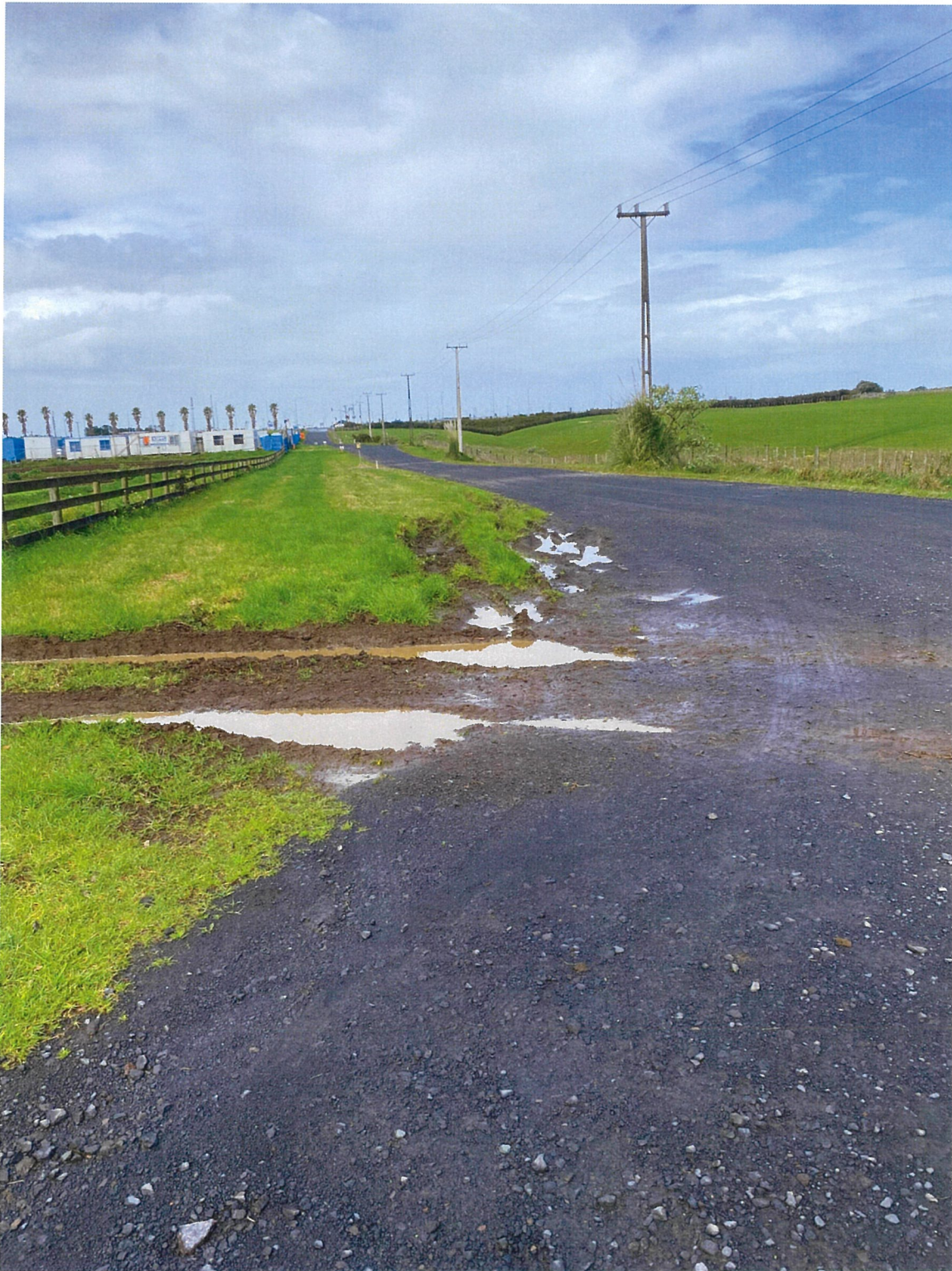
The metal surface after rain of Campana Road looking towards Puhinui Road (Date 30/08/2025)
