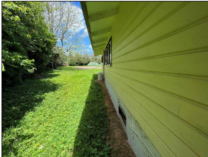
Photo 3: Exterior of the dwelling (eastern side). Cladding comprising potential asbestos containing material (PACM).
