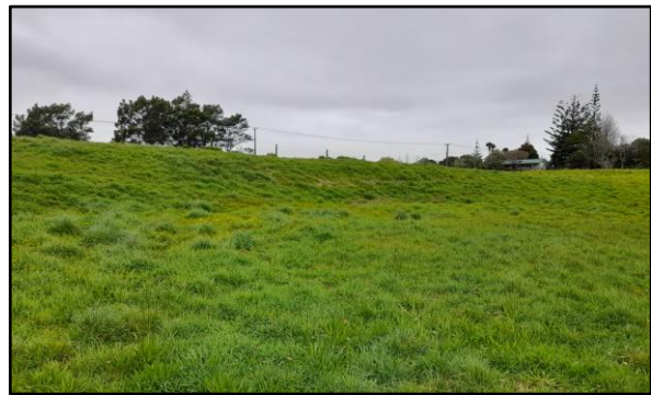
Photo 2: Western head scarp facing southeast.
