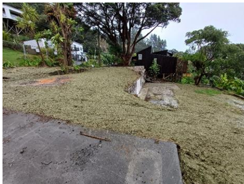
Concrete wall and slab left in place as acting as retaining (grass is still to establish)
